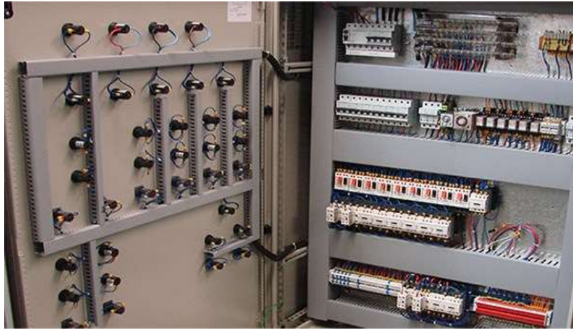
Figura 2. 1 Tablero de control
